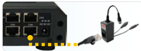
On-board RJ45 sockets and camera balun
