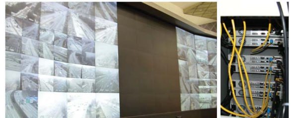
Comart System HDS device is used for monitoring of The Korea Highway Corporation Gyeonggi-do and Gyeonbuk area Monitoring Centre.
